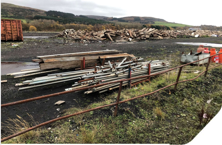
Plate 13: View of site, showing a cabin and a pile of concrete blocks (removed rail track footings) in the background, and metal rods, timber and gas cylinders in the foreground facing SE
