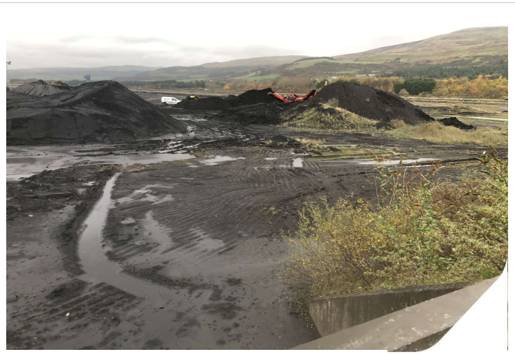
Plate 32: On going coal clearance work (in the background) at the time of visit facing N
