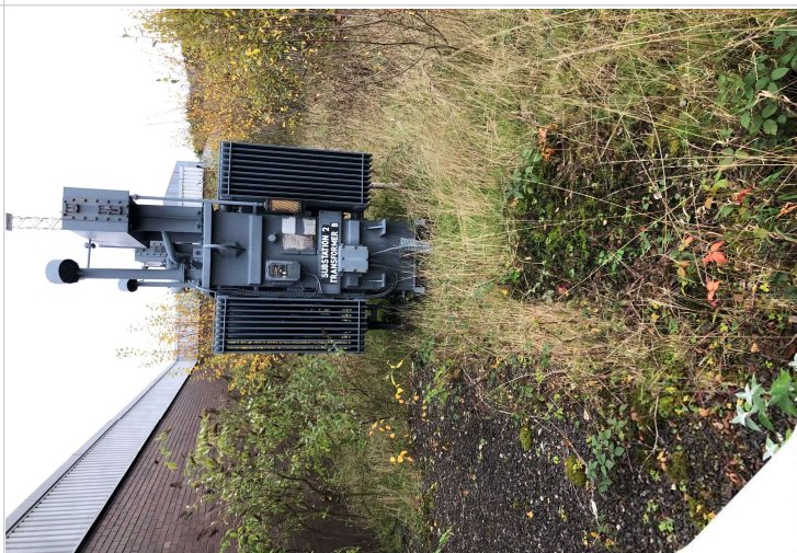
Plate 29: Transformers (sub-station) facing NE
